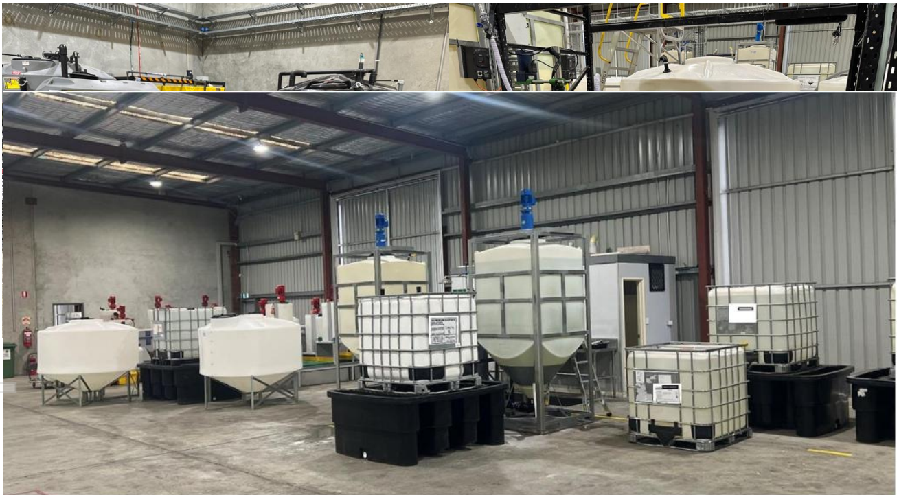
Figure 1. The HiPurA pilot plant: note the filtration units still in wrappers.
